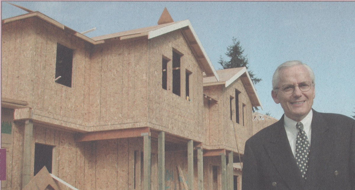
President Argue at one of the new duplexes. These units are the first buildings constructed under the college's new Master Plan.
