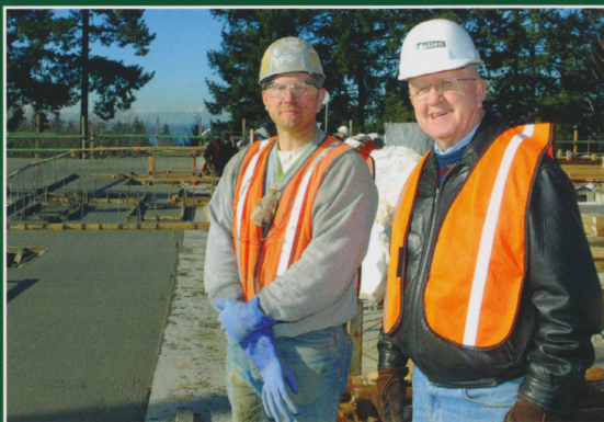
Reunion on the Roof for Alum and Professor Eric Bell of Sellen Construction chatted with his former professor, Dr. LeRoy Johnson, on the roof of the HSC.
