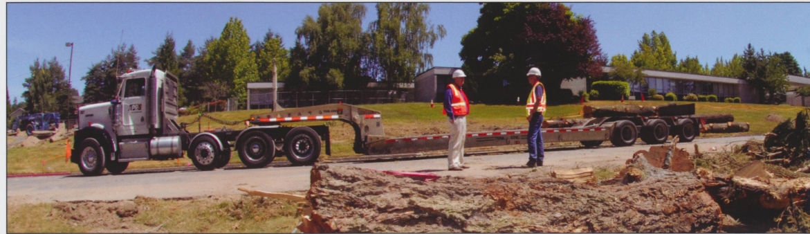
CONSTRUCTION OF THE NEW HEALTH AND SCIENCES CENTER BEGAN IN EARLY JULY. SEE PAGES 8-9.
