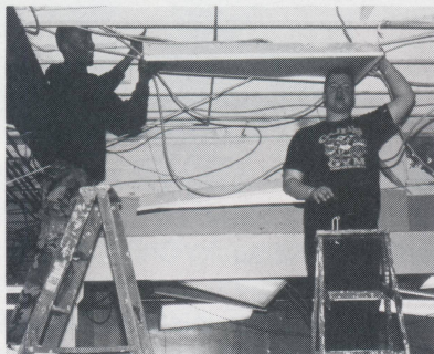
James Boyd and Stuart Curry helped install some lights at the church.
