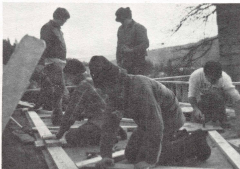
Chuck Foster (foreground), Gospel Team coordinator and group leader for the Bingen project, tackles roof job with other students.
